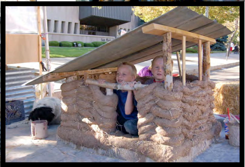
A Natural Building Cob Construction Dog House built in one day by festival attendees.
